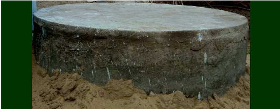
Provision for Septic Tank in all 17 Permanent Houses will enable the families gain further entitlements from the Government
